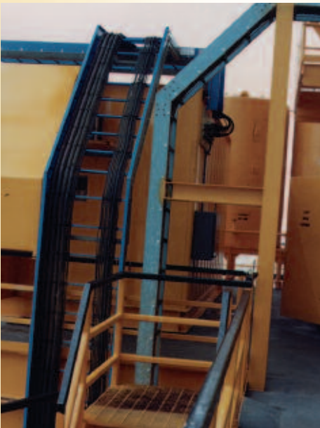
Vertical cable dropout from horizontal run
